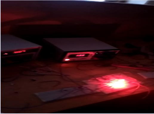
Battery charging system
